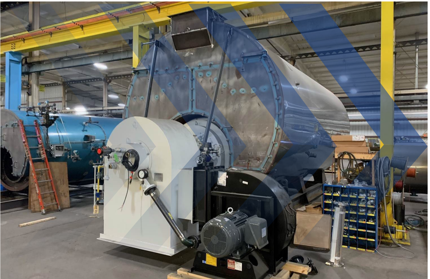
500HP firetube boiler with SPEC-COM Hydrogen burner
